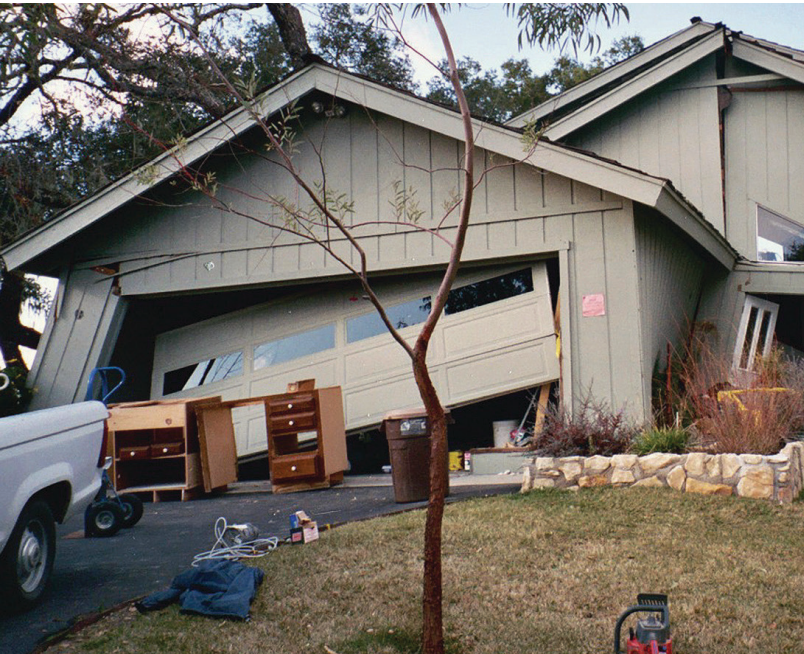
(ABOVE) ATASCADERO, CA JANUARY 25, 2004 -- THIS HOME SLID TWO FEET OFF ITS FOUNDATION DUE TO THE 6.5 SAN SIMEON EARTHQUAKE. PHOTO BY DANE GOLDEN / FEMA NEWS PHOTO
