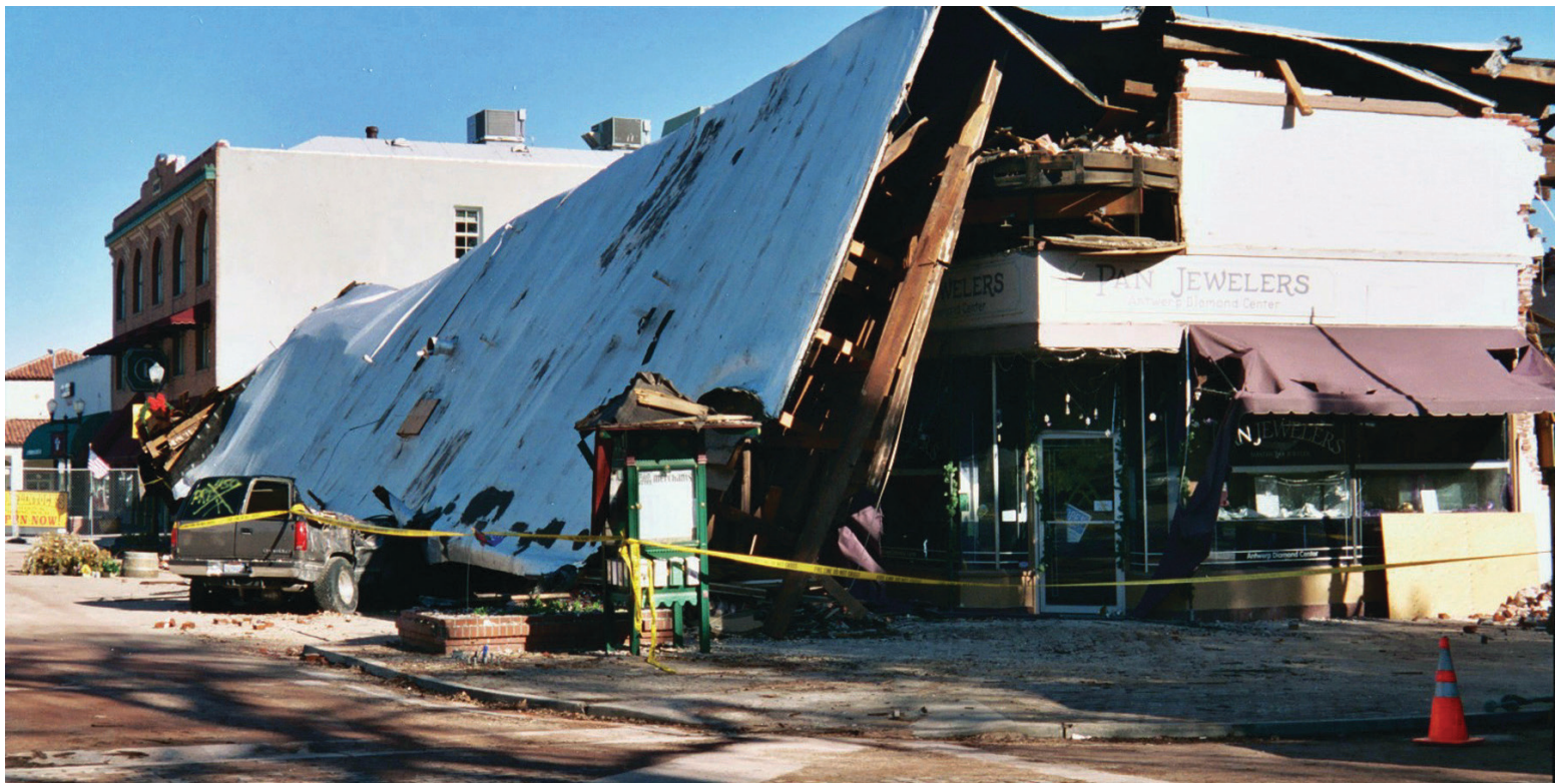
(ABOVE) PASO ROBLES, CA JANUARY 25, 2004 HISTORIC STRUCTURES AND A VEHICLE DAMAGED IN DOWNTOWN PASO ROBLES IN THE 6.5 SAN SIMEON EARTHQUAKE. PHOTO BY DANE GOLDEN / FEMA NEWS PHOTO
